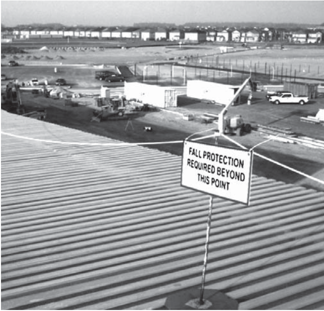
Warning barrier with sign
