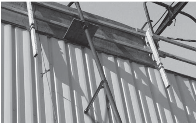
Asphalt pipe at roof level
