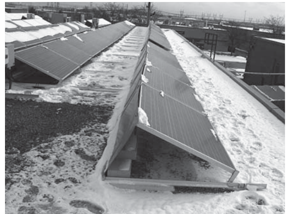
Ballasted PV system
