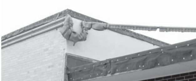
Powerline with protective insulation
